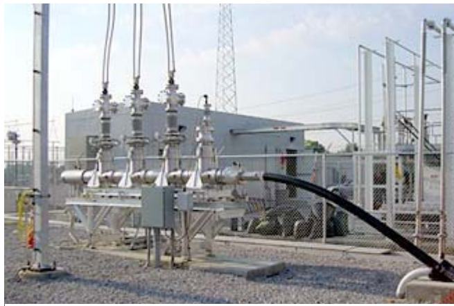
Bixby substation, Columbus, Ohio Photo from www.supercables.com/Demonstration/demo.html
