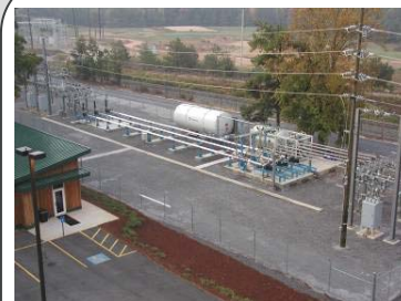
Carrollton, 30-m 6 Yrs Operation 12.47 kV, 1.25 kA, Single-Phase cables (Southwire, 2008)
